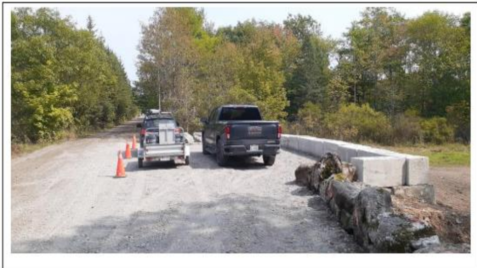
Photo 8: Phase III barricade/crib that now acts as an ATV parking area along EOTA trail. Public Safety is first and foremost. This park was purchased with the explicit purpose of owning and operating a safe recreation and nature park.
