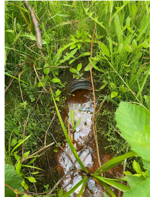
3inch drainage pipe
